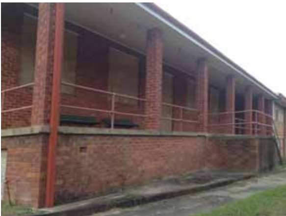
PICTURE 21 – RECREATIONAL HALL (ITEM 25)
